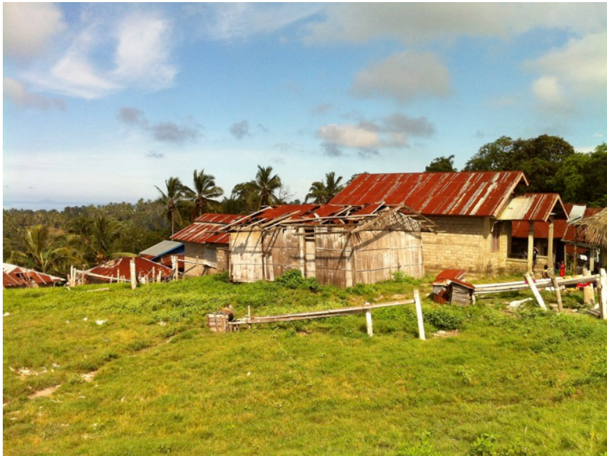
3. Houses became damaged by the volcanic dust, particularly roofs, which oxidized quickly. Cawalo village, 2014.
